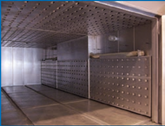
Interior Supply and Return Ducts with Interior Lighting
